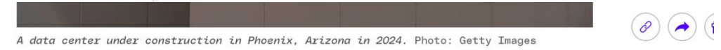
A data center under construction in Phoenix, Arizona in 2024. Photo: Getty Images
